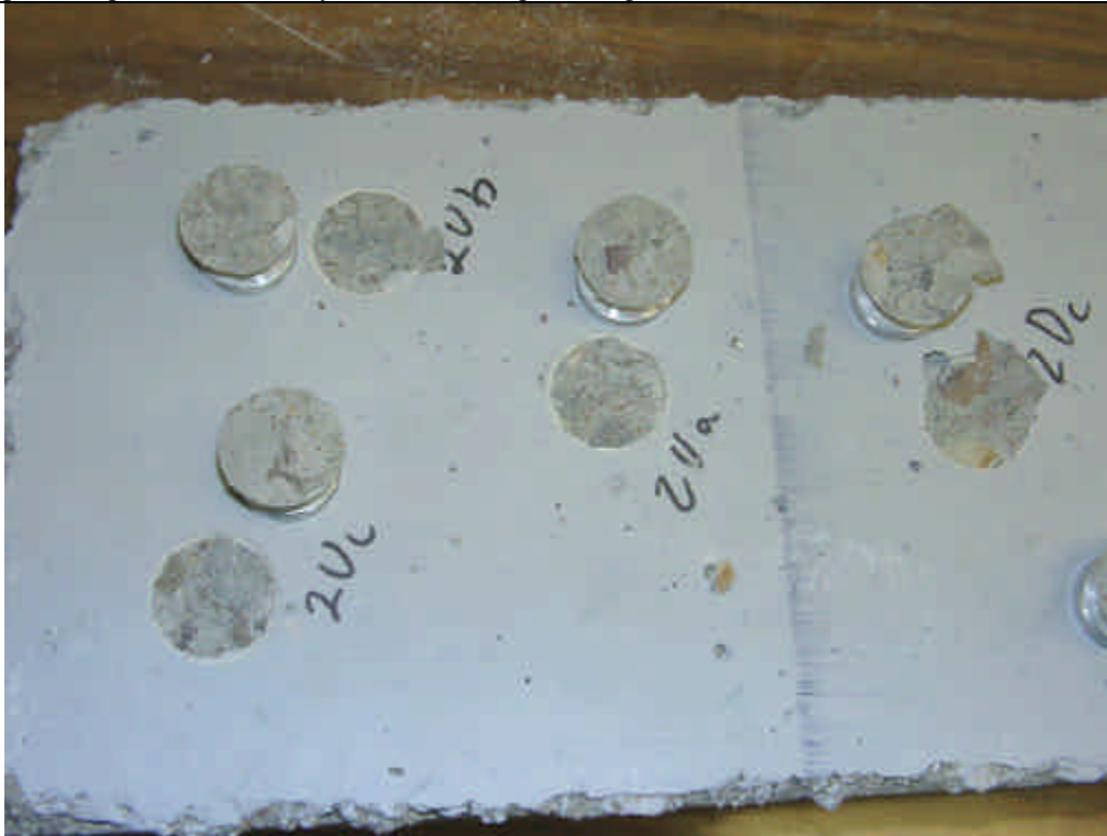
Figure 4 View of sample 2 (untreated) after dolly adhesion testing showing cohesive failure of the concrete substrate.
