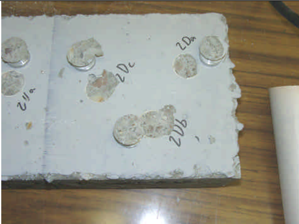
Figure 3 View of sample 2 (degreased) after dolly adhesion testing showing cohesive failure of the concrete substrate.
